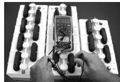
Fig.2 - OCV being verified with a voltmeter
